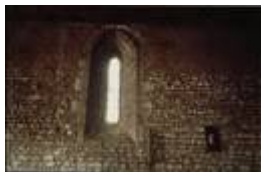
125. Dragey. The north wall of the nave (inside). The inner plaster of the side walls was scraped by the villagers to show the opus spicatum (fishbone masonry), at the request of abbot Pierre Danguy, pastor of the church between 1954 and 1974. The opus spicatum - with lines of schist plates arranged horizontally - attests the church was built in the 11 th century and early 12 th century. The long bay with a deep splay is from the 13 th century. Photo by Alain Dermigny. [Alain_067]
