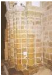
149. Genêts. The Romanesque transept crossing. One of the tower piers. Two sides have a flat non-molded surface. On the other two sides, the arches are received by two attached twin columns on a backwall. In one corner, an attached column receives the spring of one arris of the vault. The carved basket capitals are topped by a thick square abacus. The square bases are topped by a double torus. The pier itself rests on a broader square base. The other three pillars are perfectly symmetrical to this one. Photo by Claude Rayon. [Claude_45]
